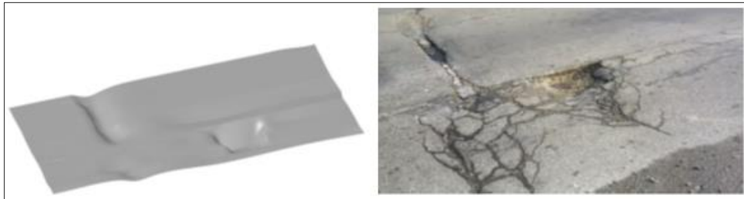
Figure 4. Holes on the road surface and the 3D view produced by the system
