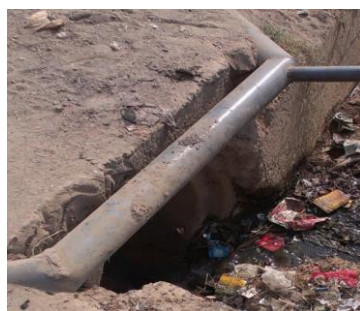
(a) Sharp edges in distribution pipes
