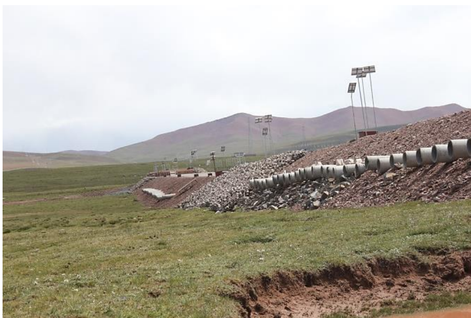
Figure 1. Ventilation ducts, seen as a row of concrete pipes in the earthen dam, are embedded in a railroad embankment to cool the underlying permafrost in Qinghai-Tibet Railway. Air enters from one end (inlet) and leaves from the other end (outlet)
