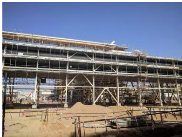
Figure 4. Photograph of the pipe rack module under consideration
