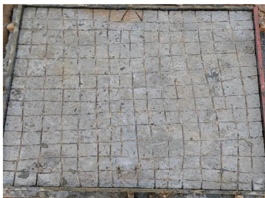
Figure 7. Preparing the surface of the substrate layer of the slab specimen (made groves)
