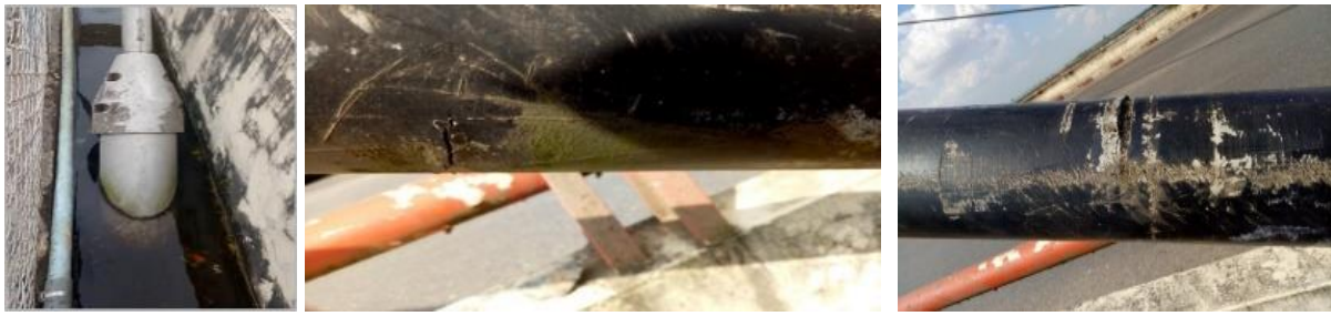
Figure 7. Poorly drain condition and cable anchor zone in damp condition and cracks and damage in sheathing of cable3 D/S in December 2018
