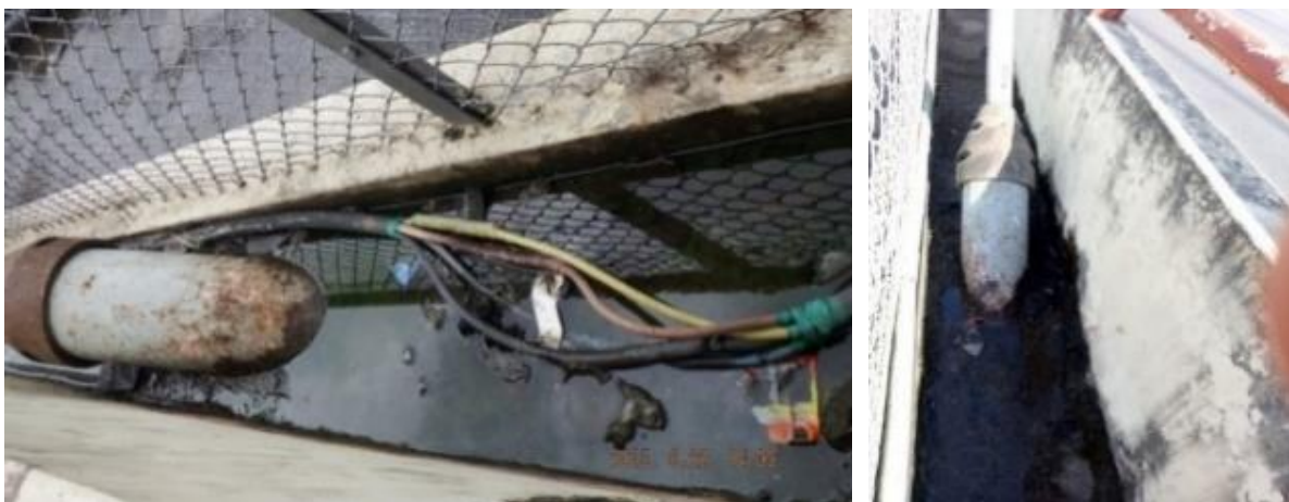
Figure 6. Drainage blockage in cable anchorage zones (MOC, 2015)
