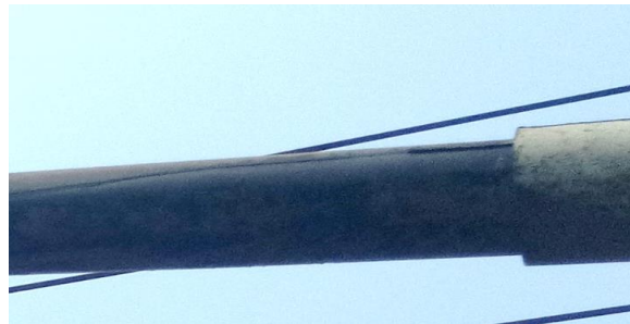
Figure 9. Cracks in sheathing of cable30 D/S in August 2019
