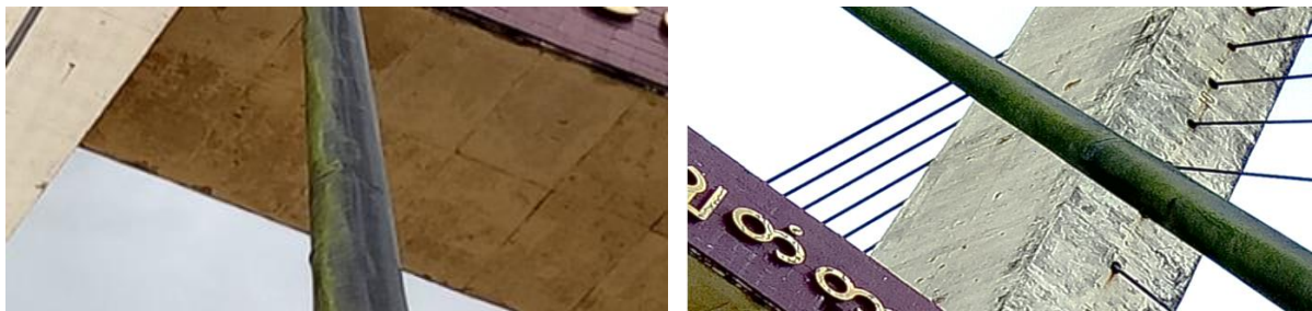
Figure 10. Water stains on lower portion and cracks in sheathing of cable33 D/S
