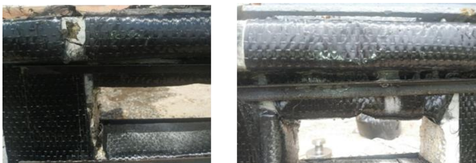
Figure 6. Typical failure mode observed for repaired beams
