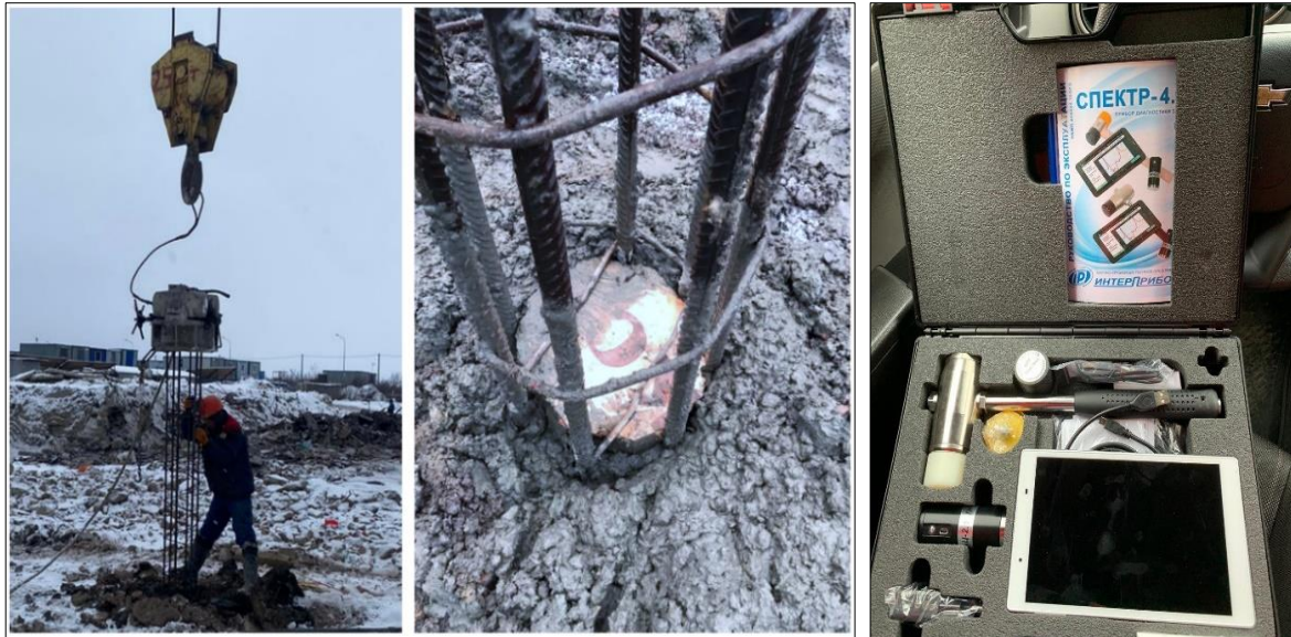
Figure 6. Construction of piles with defects
