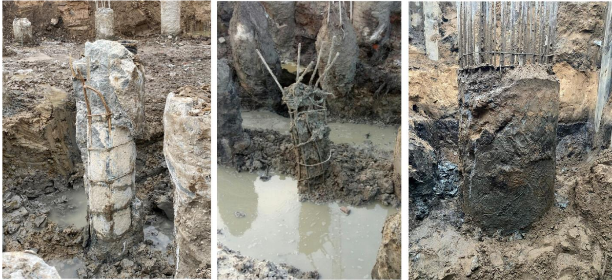
Figure 1. Common defects in cast-in-place piles: necking, washout, and soil inclusion (from left to right)
