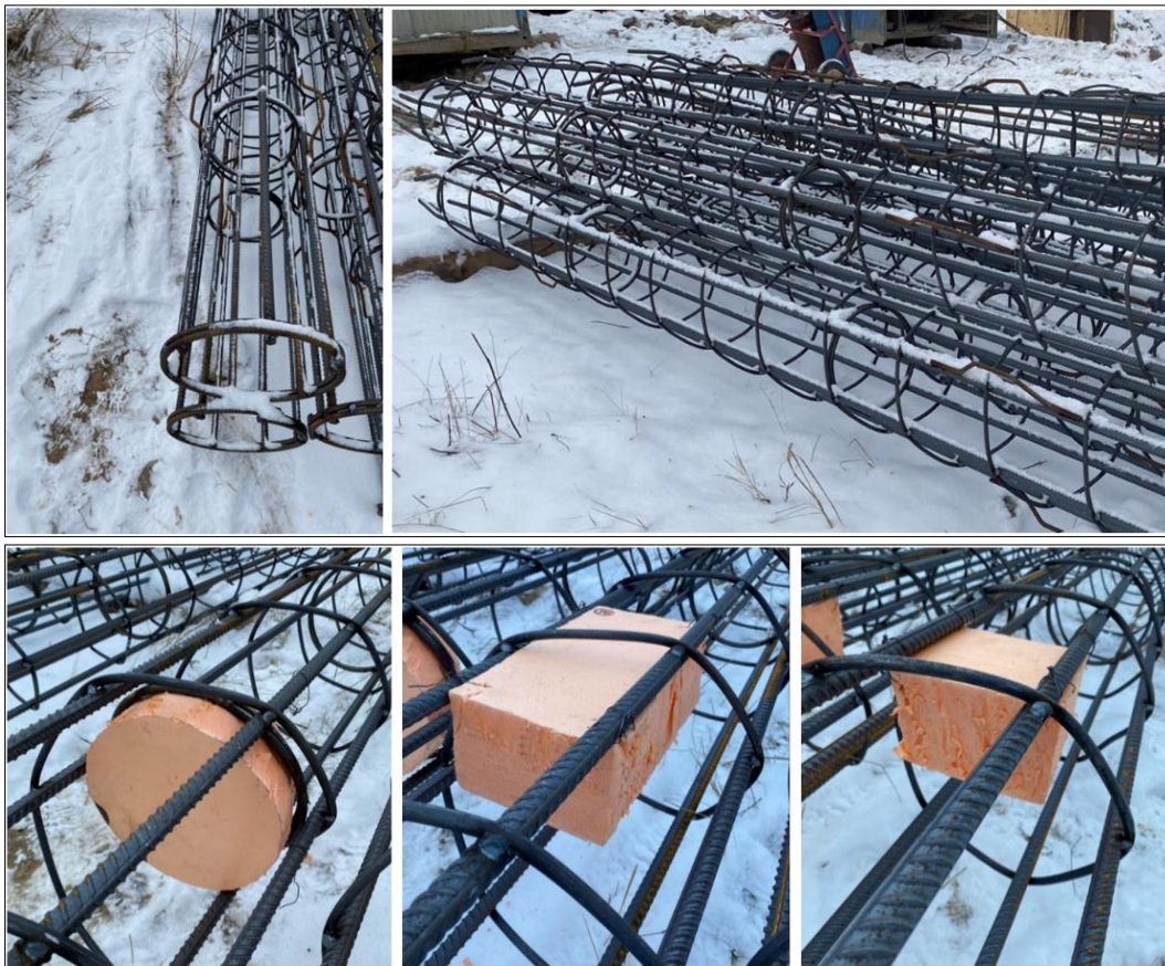
Figure 5. Reinforcement cages before (1 st row) and after (2 nd row) the installation of defects
