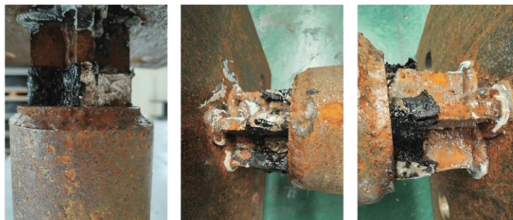
(b) High-temperature-induced melting of unbonded materials
