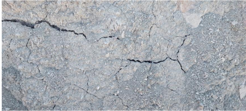
Figure 1. The clay crack in situ
